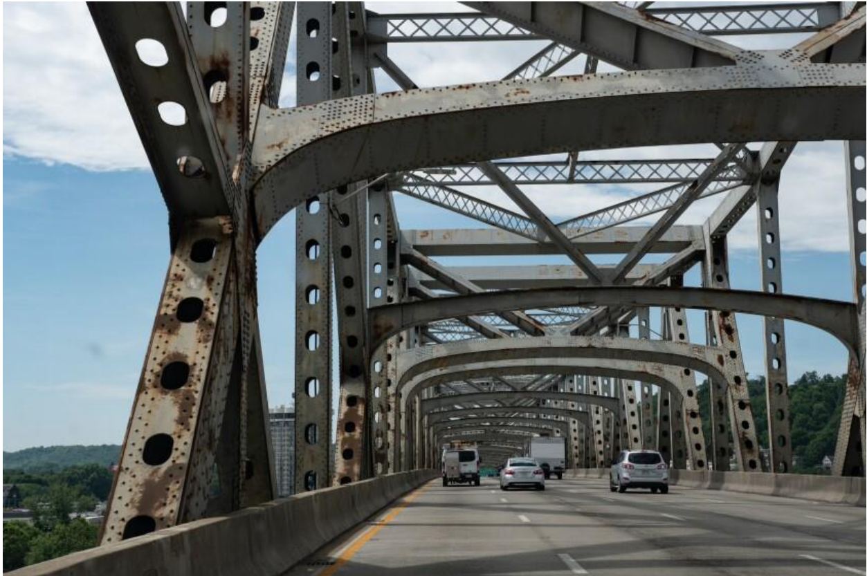
Maintenance of the Brent Spence Bridge has fallen behind and upgrades have been nonexistent. AdobeStock
