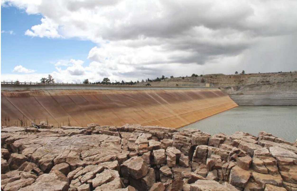
The El Vado Dam in New Mexico's steel faceplates need replacement or repair. Bureau of Reclamation
