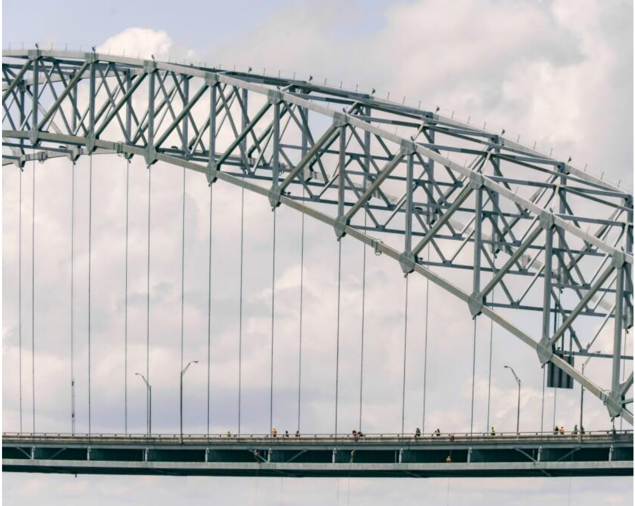
The I-40 Hernando de Soto Bridge closed on May 11 after the discovery of a cracked and almost-severed steel beam.
