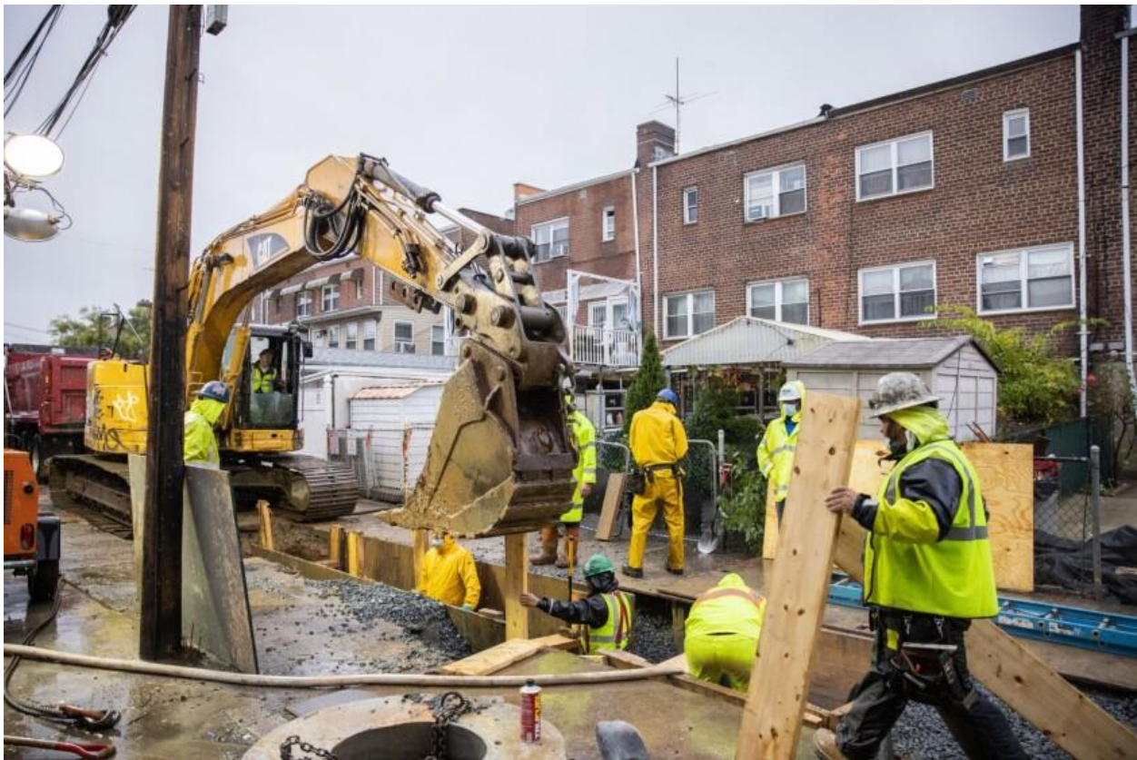
Workers on a construction site repair damage from Hurricane Ida in the East Elmhurst neighborhood in the Queens borough of New York. Bloomberg News
