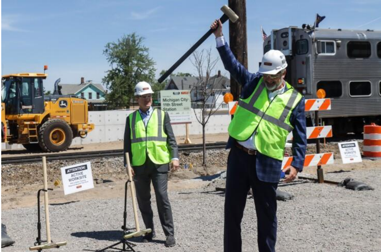
Indiana Gov. Eric Holcomb wields a hammer at a June ceremony to mark the start of construction on a second set of tracks for the South Shore Line commuter railroad. Indiana governor's office
