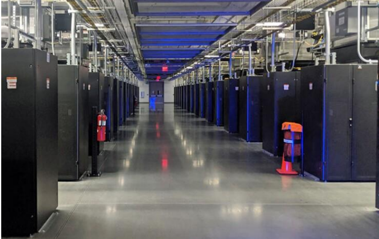
A view inside the Facebook/Meta data center in Papillion, Nebraska, when it opened in 2019. Data operations by Meta and Google parent Alphabet are driving electricity demand for the Omaha Public Power District. Omaha Public Power District
