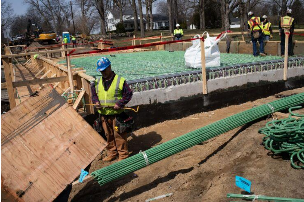
Contractors work at a Michigan Department of Transportation bridge construction site in 2022. The state is issuing $1.18 billion of bonds this week for highway construction. Bloomberg News
