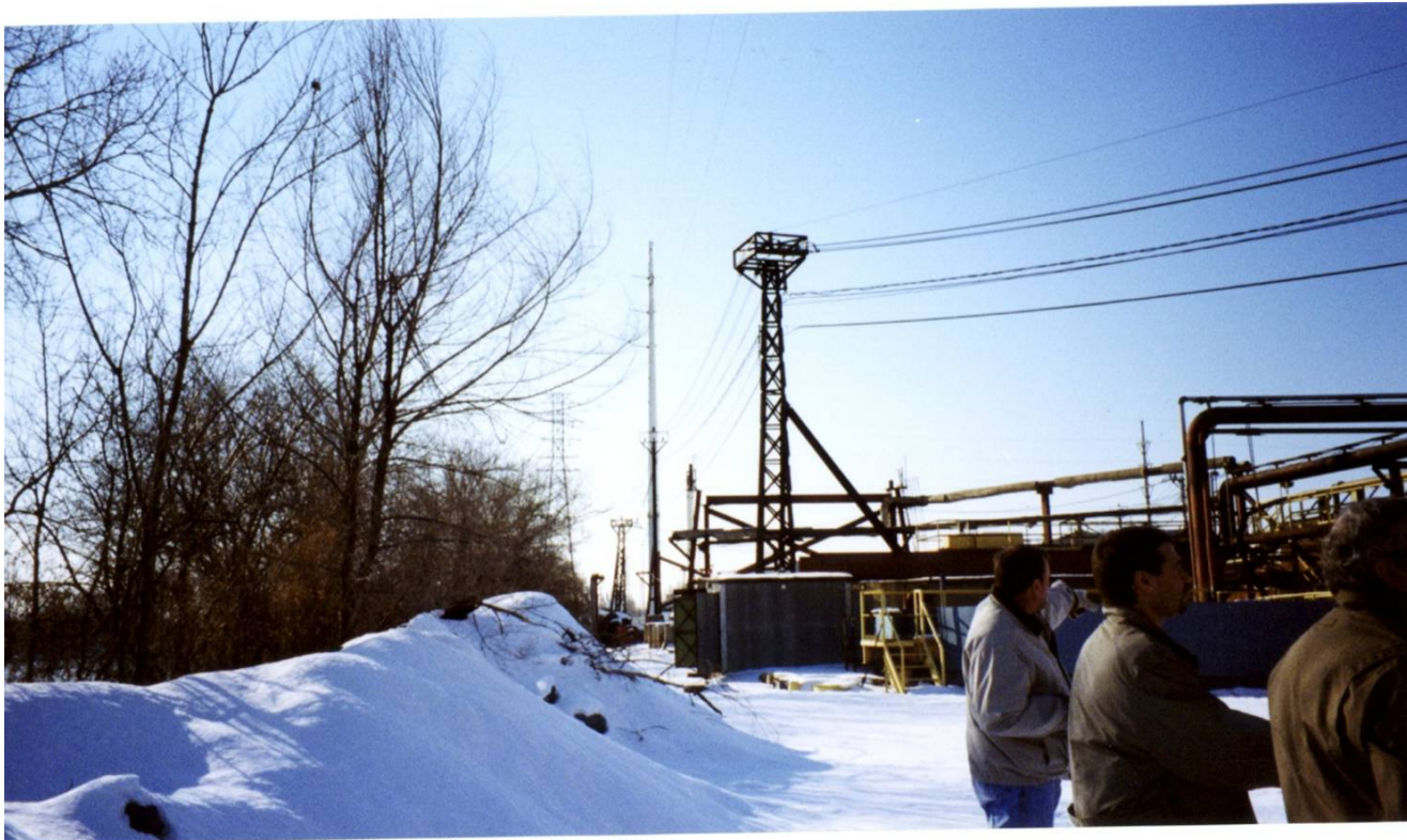
Looking west- towers that carry 138KV to Pentagon substation
