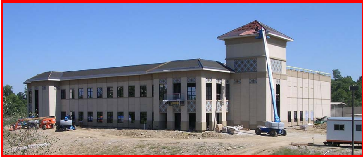
New KMBC offices under construction, looking north (top) and looking east (bottom)
