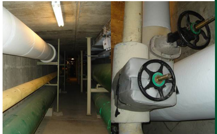
Grand Valley State University added approximately 8,000 feet of 1.5 inch steam piping installation to the main tunnel and branches underneath the campus; steam valves were also covered with insulated boots. The project is estimated to save the university approximately $187,935 every year in reduced operating costs.
